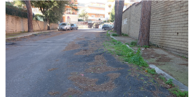
Figure 5.19. Streets with potholes and inadequate sidewalks scored 1
