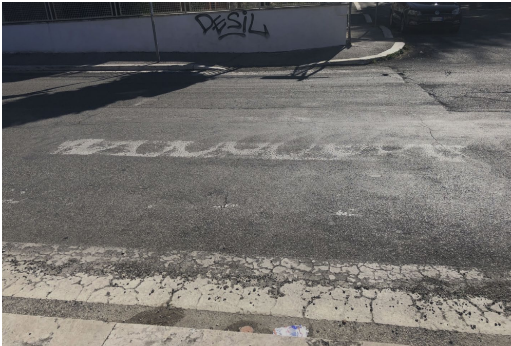
Figure 31: Via della Consolata -- lack of visible crosswalk to access the urban garden
