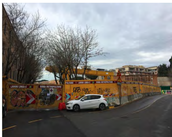
Image of the construction currently taking place in San Giovanni for the Metro C
