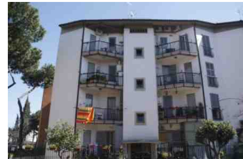
Fair: Clean exterior, possibly some street level graffiti / Medium balconies / Paint slightly worn
