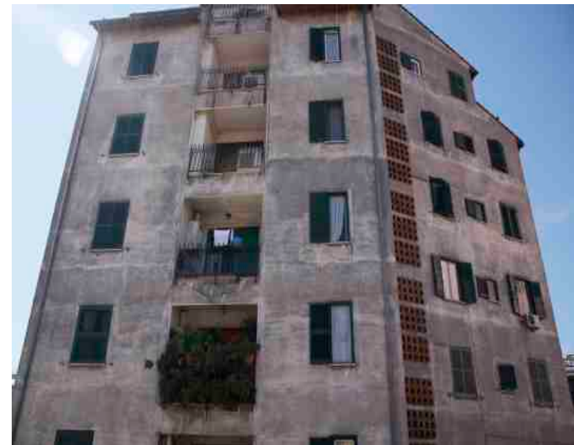
Figure 3.2 Poor Upkeep The poor upkeep of the gray INA-Casa towers on Via dei Crispolti stand out in the generally well-maintained neighborhood (Yoon 2009).
